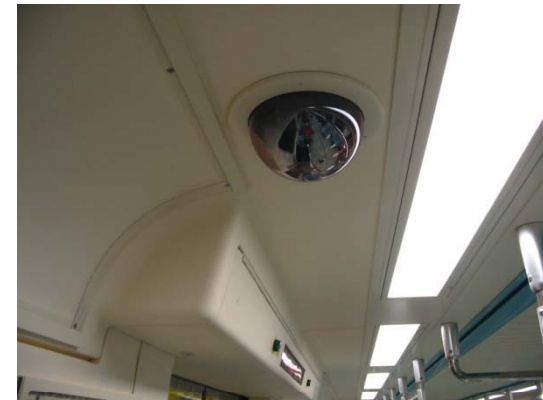
MRT Interior Camera(PTZ Control)
